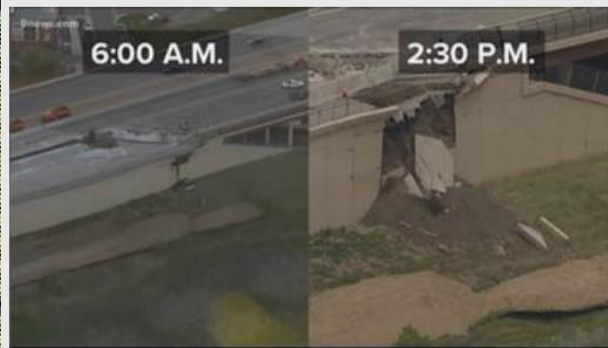
Figure 1: Highway 36 collapse over time. The cracking on the highway's surface was noticed a week prior to the incident, and was seen to be spreading the night before the complete collapse. This allowed the Colorado Department of Transportation to be prepared to re-route traffic and begin mitigation efforts.
